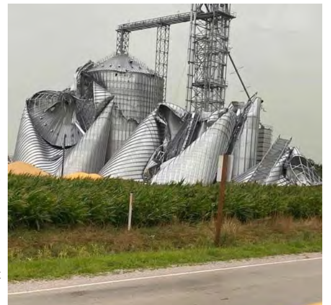
Some of the derecho’s damages. Photo courtesy of The Weather Channel.
