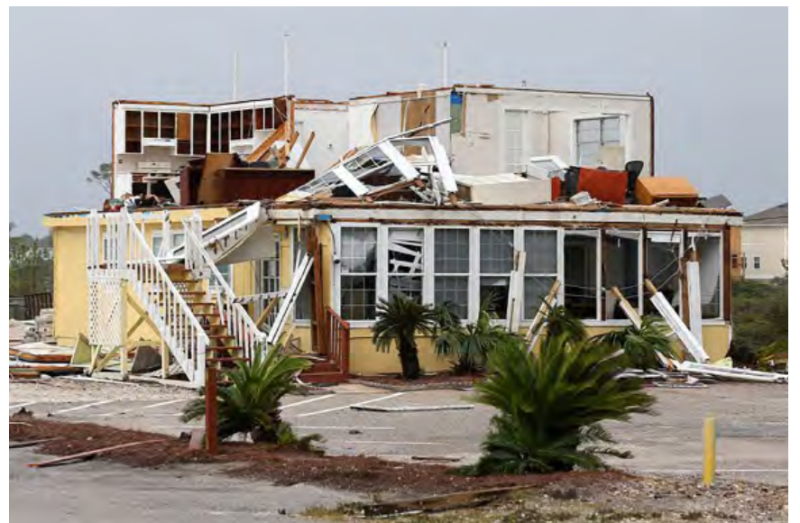
One of the many houses in Perdido Key, Florida that Hurricane Sally damaged with intense winds and 20+ inches of rain. Image Credit: REUTERS)
